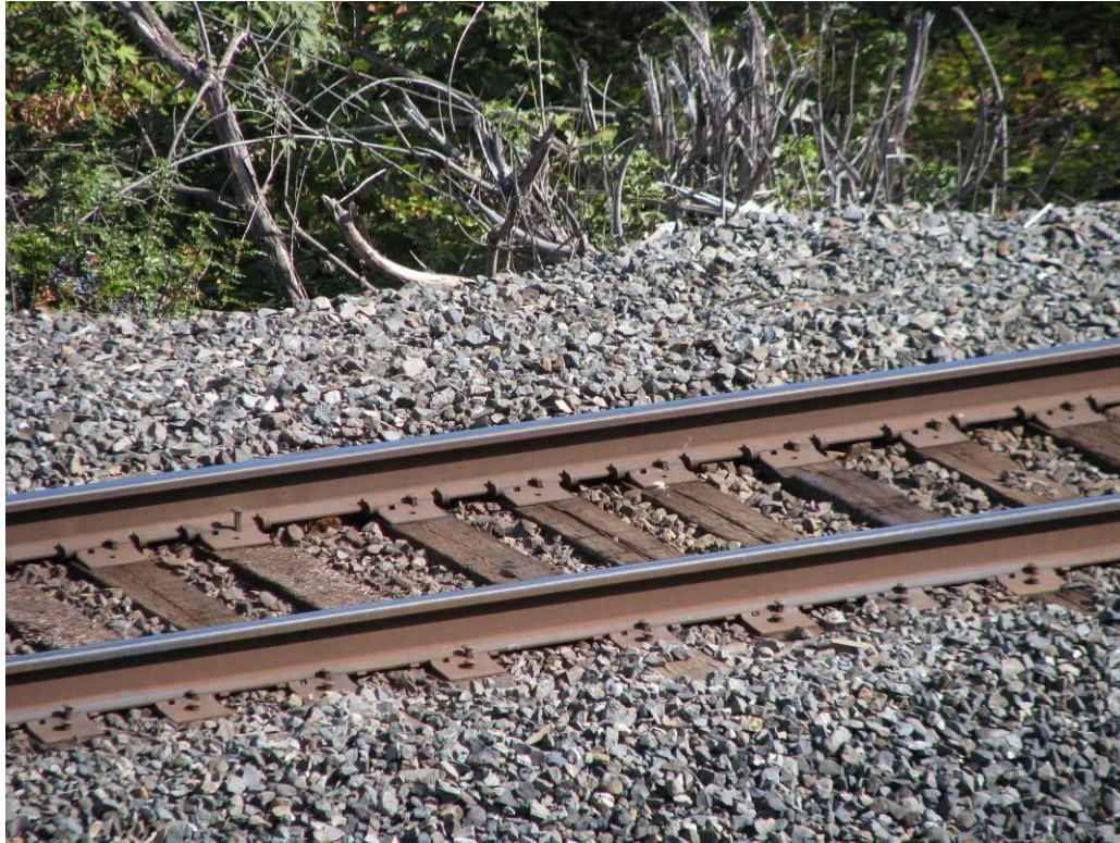
Figure 4. Detail of OR&N tracks, showing replacement steel rails, wood ties and gravel ballast, viewing north from Highway 30 overpass (AECOM 2020).
